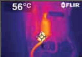
What a thermal imaging camera sees.
