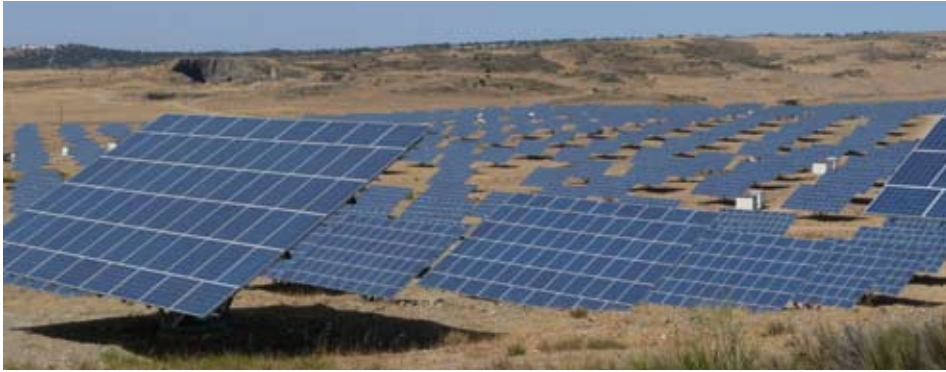
A part of the Abertura Solar Power plant.
