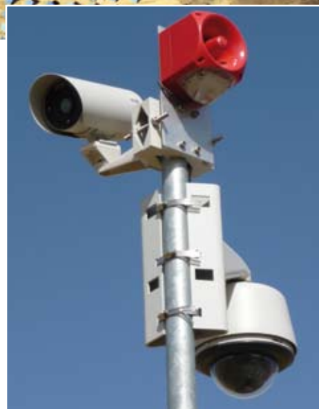
FLIR Systems SR-35 thermal imaging camera, a sound and light beacon and a CCTV dome installed at an observation point at Abertura Solar Plant.
