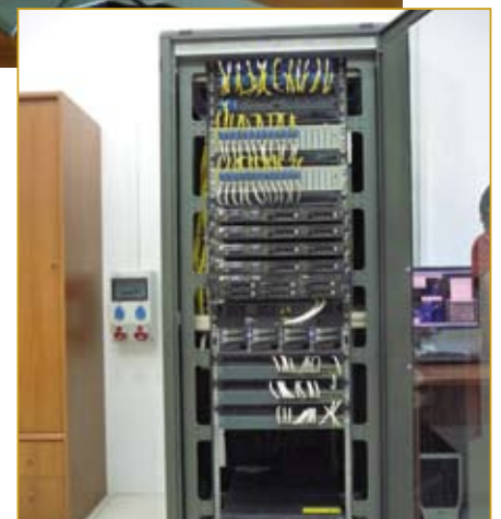
A rack in the control room converts the Fiber optic to Ethernet. It also contains the FLIR Systems Video Processing Units and the FLIR Systems Network Digital Video Recorders.
